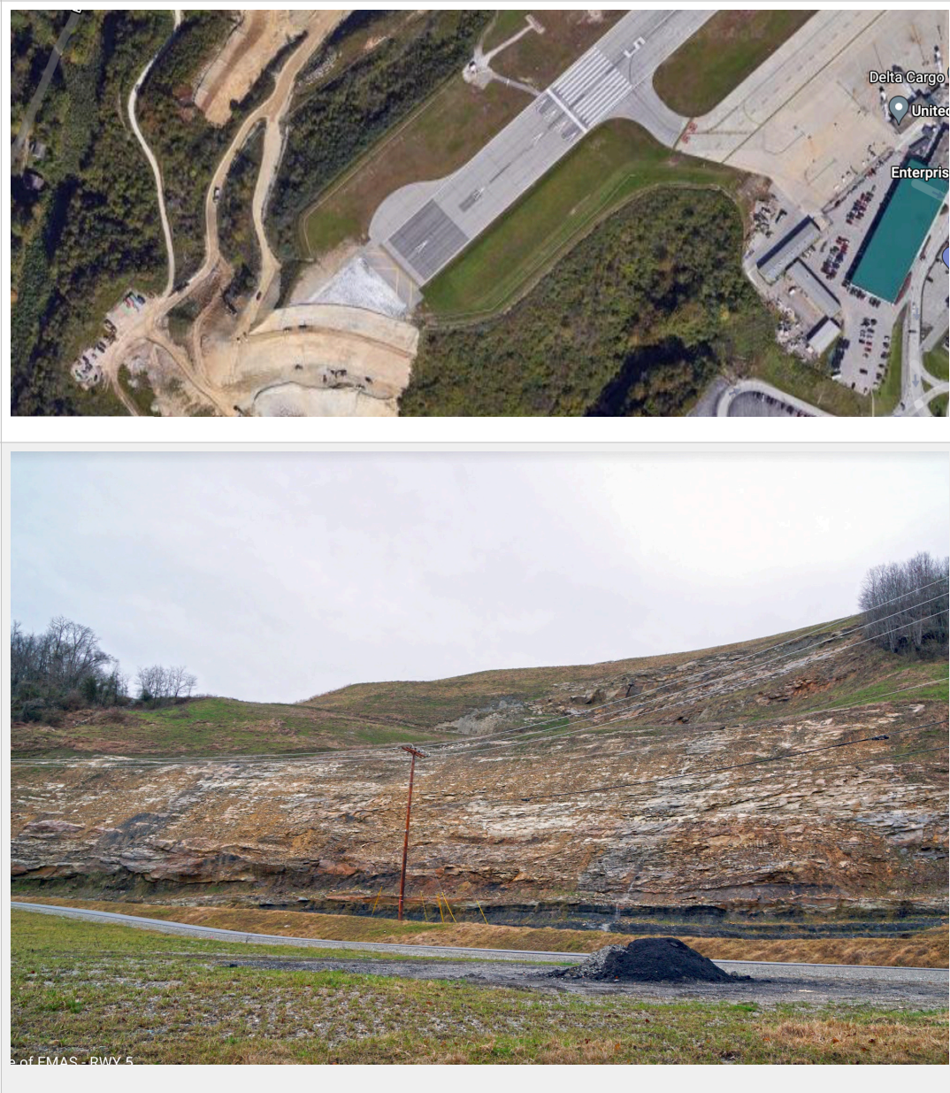
Figure 1. Charleston (West Virginia ) Airport Runway 5 end after geotechnical collapse of retention wall.
